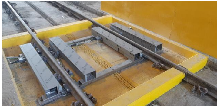
Figure 1 Wheel Measurement Equipment installed within the sand plant at Trafford Depot
